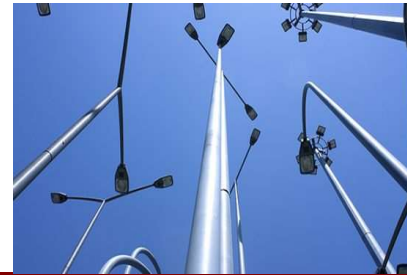
Electrical Pole Installations
